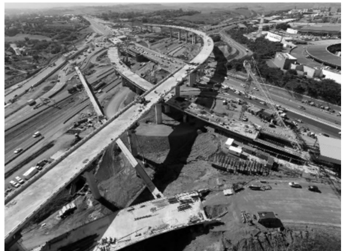
Figure 1. Aerial photo of Mt Edgecombe Interchange in March 2017 with the free flow upper level ramp in centre (SANRAL).
