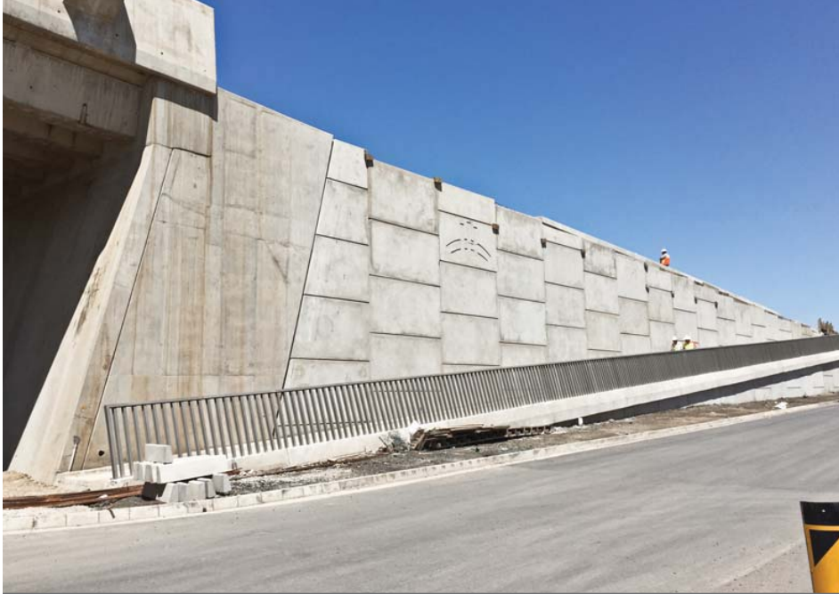
Cornubia Bridge west abutment – the abutments were slanted, which would have visually accentuated the effect of any downward settlement behind the abutment
